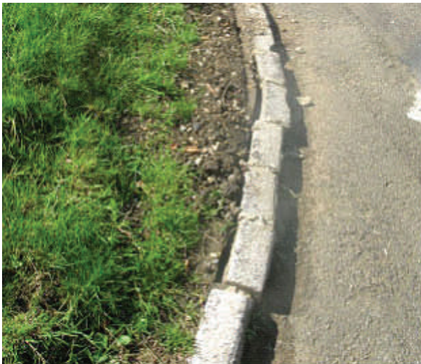
Aesthetic granite setts failing due heavy vehicles over-riding the kerb
