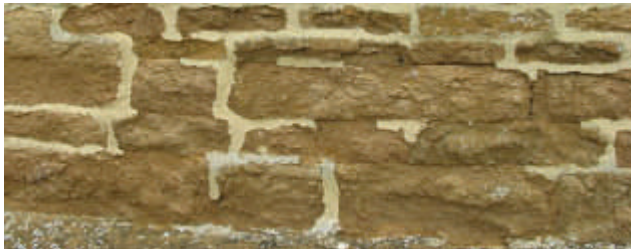
Stone decay due partially to cement mortar
