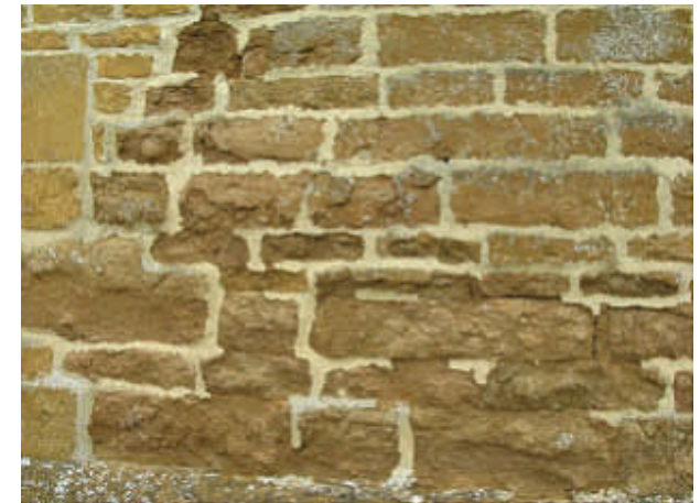
Damp created by a build-up of vegetation and soil behind this wall can eat away at the soft ironstone
