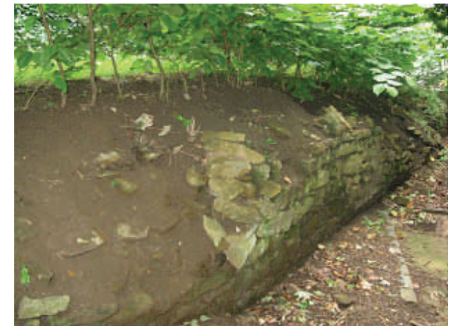
The failing retaining wall on the main road
